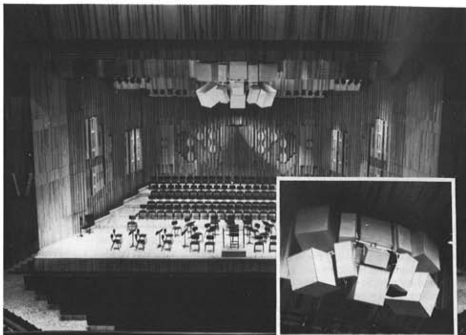
Installation at the Barbican Concert Hall, City of London. The system has since been hand-painted to match existing wood panelling.
